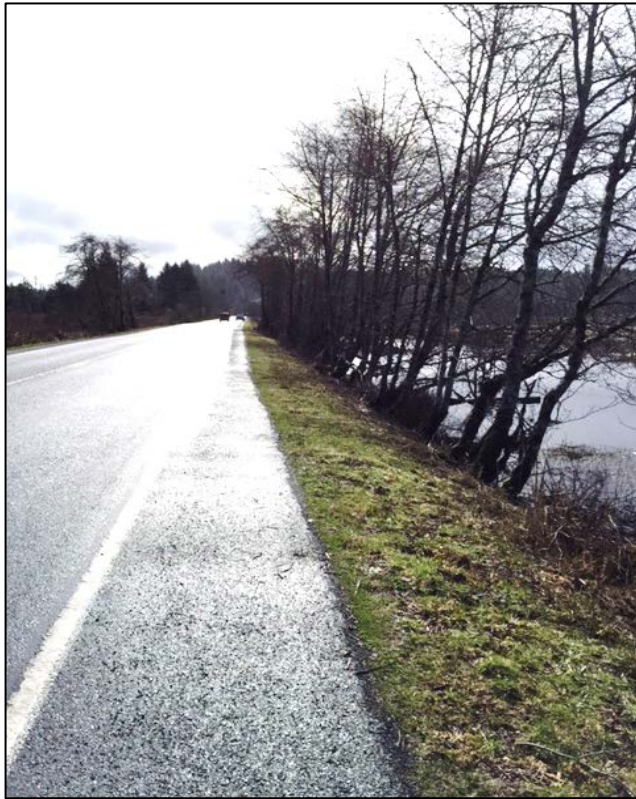
Photo 13. Proposed raw water pipeline alignment under eastbound lane and shoulder of North Beaver Creek Road. Looking east.
