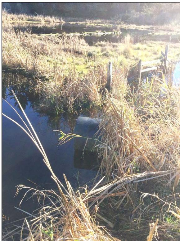
Photo 15. Beaver Creek west of North Beaver Creek Road near proposed backwash outfall. Note 36" culvert provides cross drainage beneath the road.
