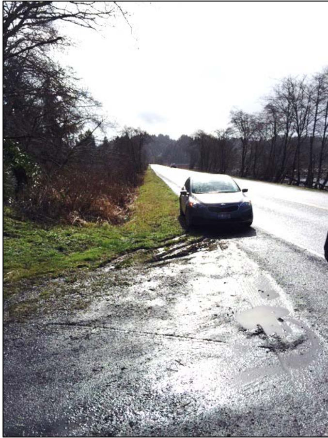
Photo 8. Proposed raw water pipeline alignment under eastbound lane of North Beaver Creek Road. Looking south.
