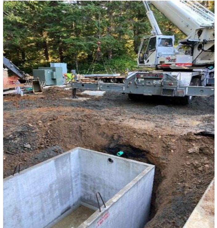
View of the precast sanitary holding tank installation north of the Backwash Basin:
