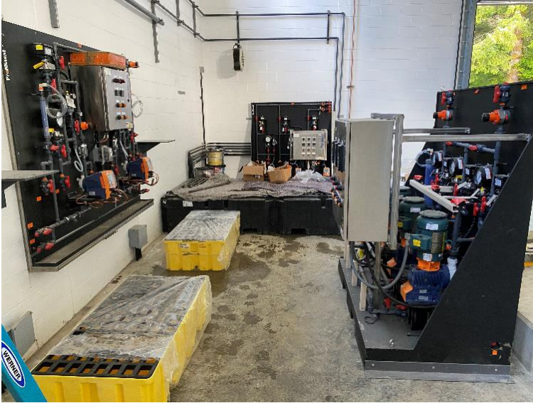
Finished water feed panels:
