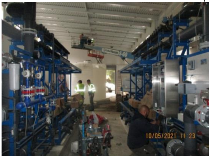
WTP Filtration Skids:
