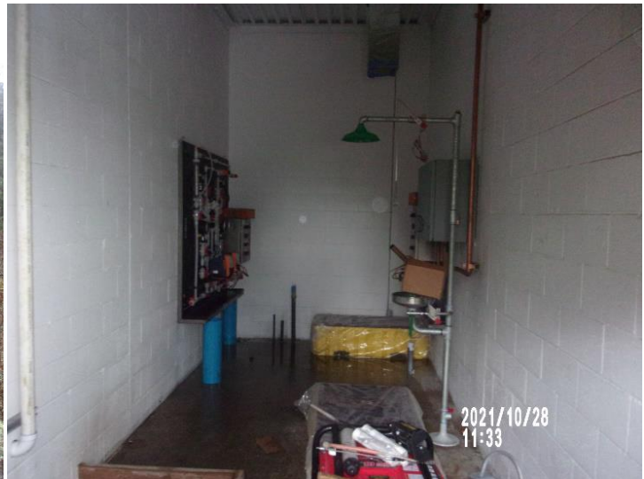
View of the mechanical room of the RW Intake Building:
