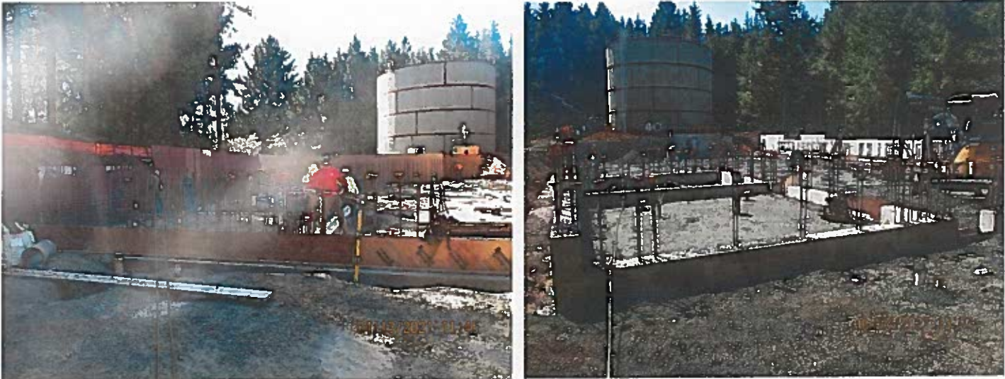
Membrane Building Construction with Clearwell in the background and Backwash Basin to the left:
