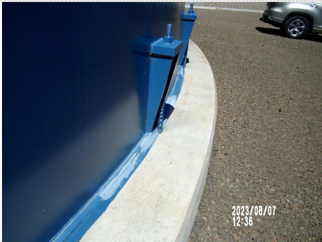
Peeling along Clearwell 1
