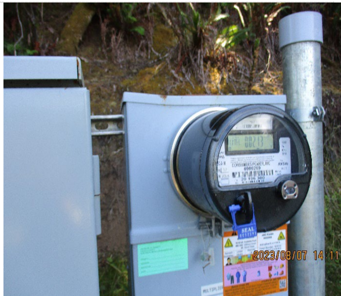
Meter damaged at Intake Site
