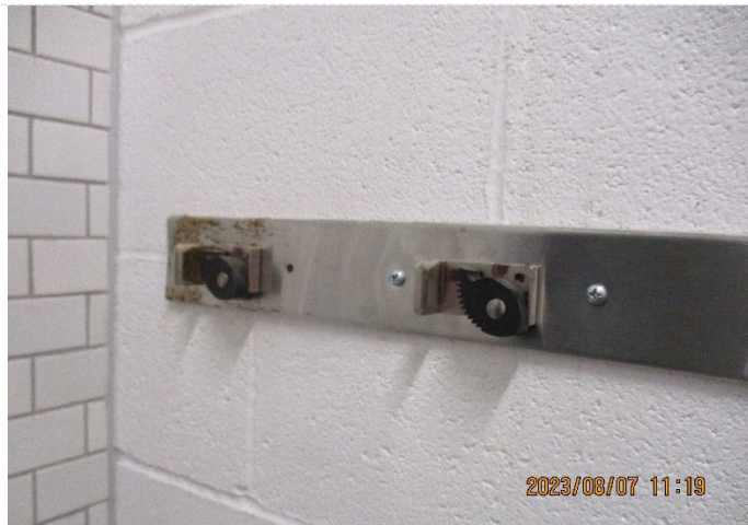
Rust observed on mop and broom holder in Janitor Room
