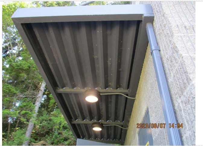
Stormwater leaking between canopy and building
