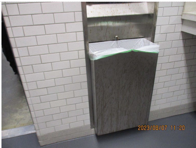
Rusting observed on the paper towel holder and garbage can
