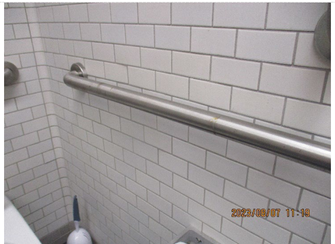
Rust observed on the bar in the bathroom
