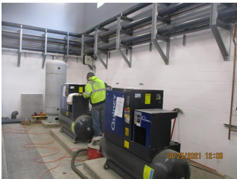
Air Compressors/Treatment Building:
