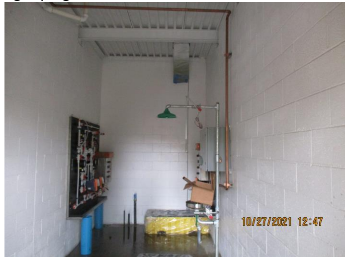
Beaver Creek Intake, Pre-Treatment Room:
