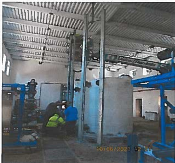
WTP Mixing Tanks:
