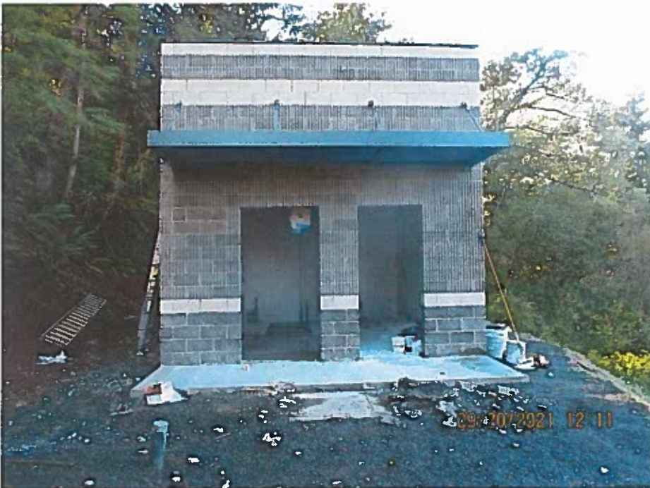
Intake Electrical Building:
