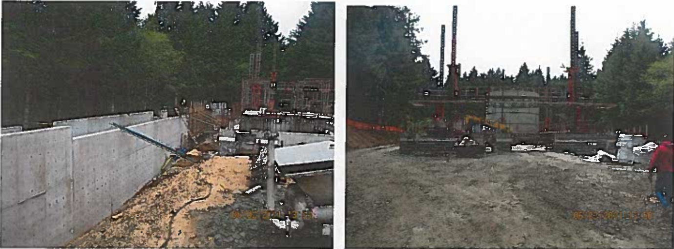
Membrane Building Construction with Clearwell in the background and Backwash Basin to the left:
