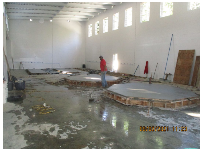
Interior Membrane Building:
