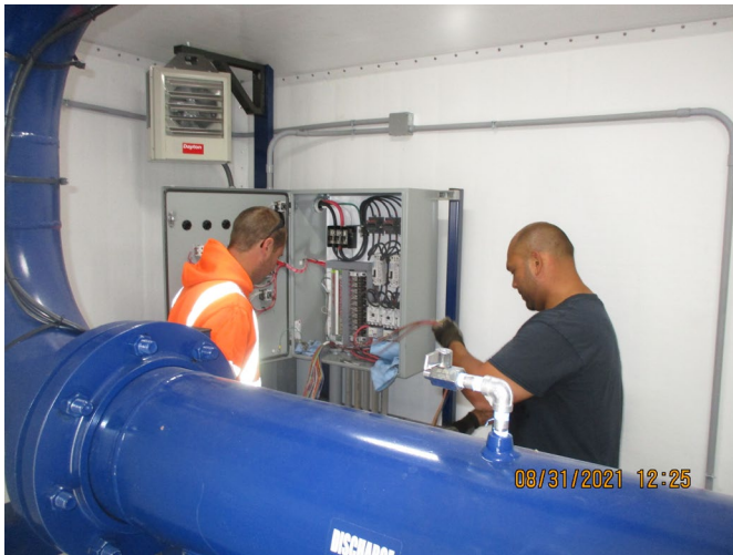
Interior view of the 123 rd Street Pump Station:
