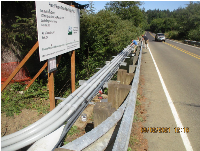
Pipe gallery across Beaver Creek Bridge:
