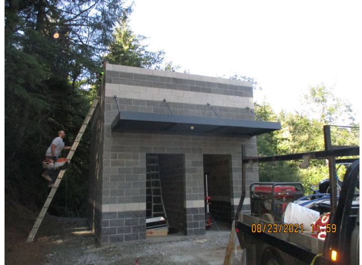
Intake Electrical Building:
