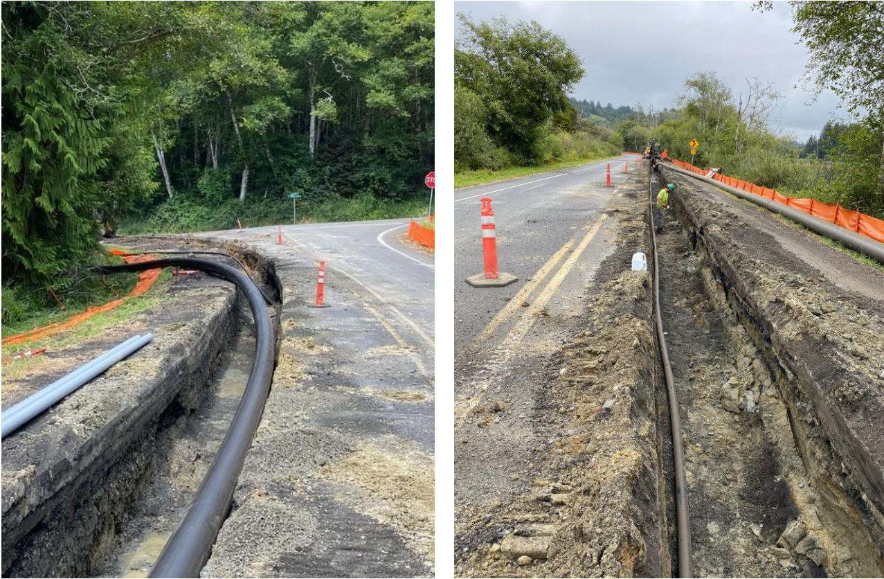
Beaver Creek Source Water Project, Raw Water pipeline installation along Beaver Creek Road:
