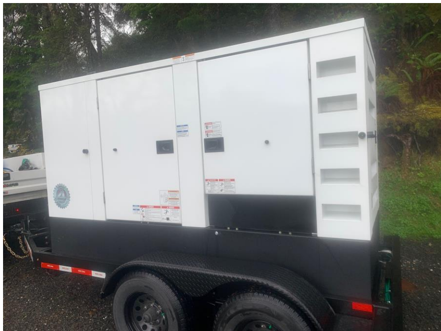
Emergency Standby Generator:
